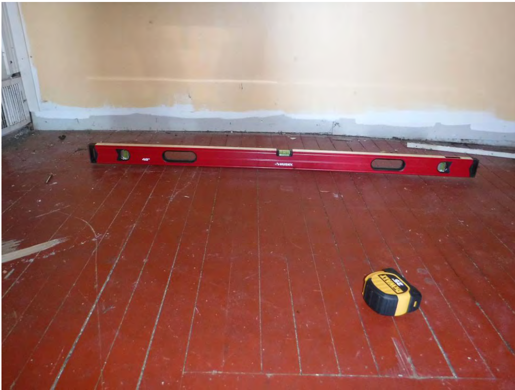
Photograph 12: Second floor at building center with high point (slope east and west).
