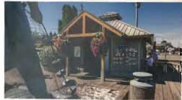
Construction begins Tuesday (Sept. 22) on the new Gig Harbor Welcome Plaza. It's a $2.5 million project in Skansie Brothers Park in downtown Gig Harbor. Andrew Blomquist / blomquist@news11.com
