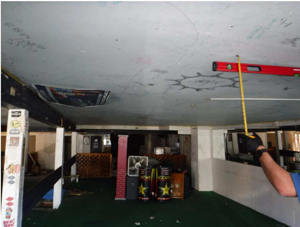
Photograph 11: Underside of second floor with slope toward exterior of 12-inch per 1-foot.
